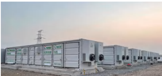
Xinyi Hydrogen Project ZSCB-6535/10kV Dry Type Rectifier Transformer
