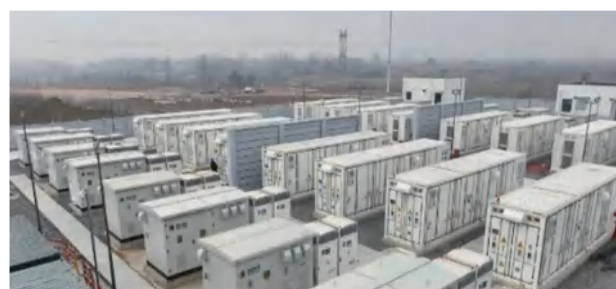
Hubei Gaoqiao 50MW/100MWh Energy Storage Project SC(B)-3450/10kV Cast Resin Dry Type Transformer
